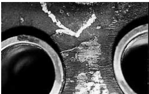
Radial crack at fire tube.
