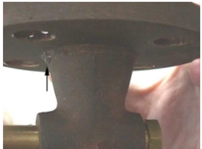
Close-up view of a gauge glass cock showing water dripping through the fillet where the flange is attached.
