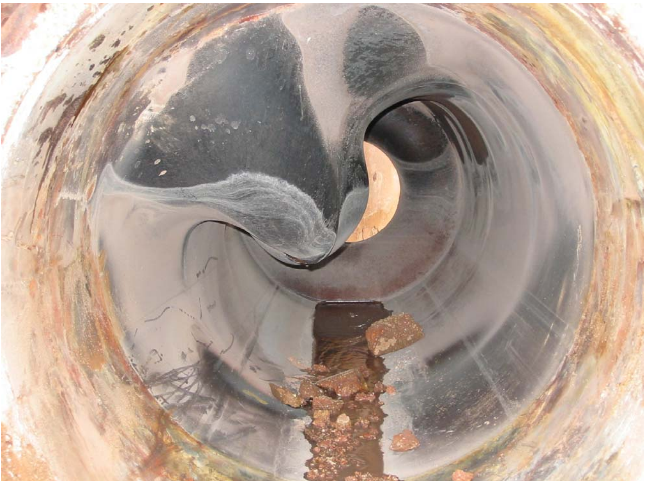
Furnace from the burner end
