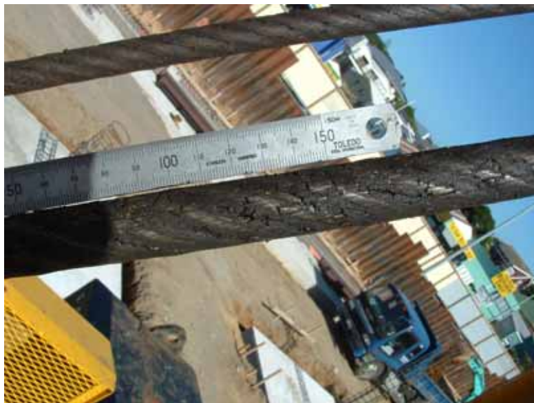
Crane luffing rope
