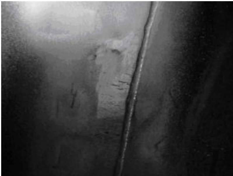
Typical cracking initially seen with MPI
