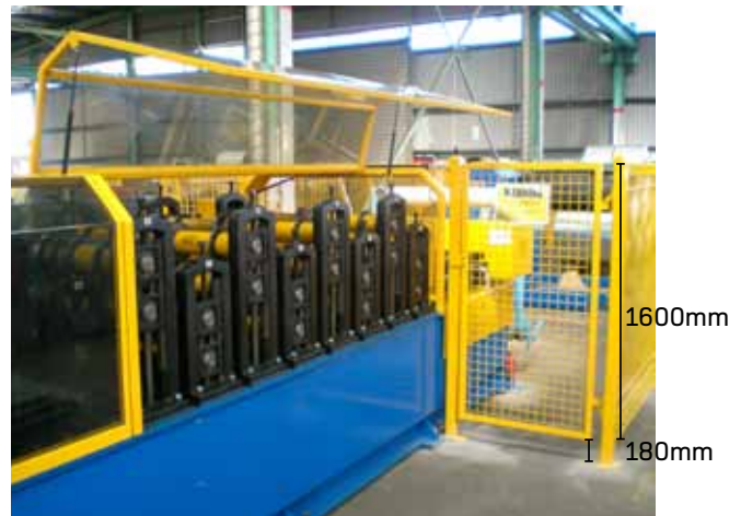
An interlock guard on a roll former.
